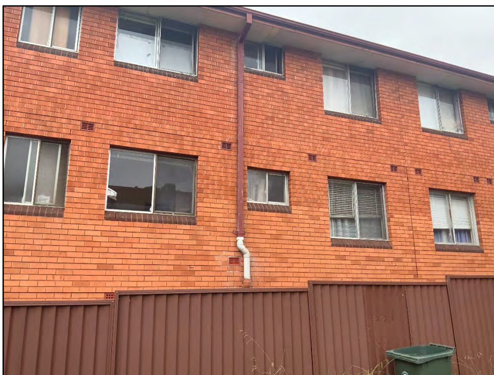
Figure 28: Interface of the subject site and the adjoining residential flat building to the south
